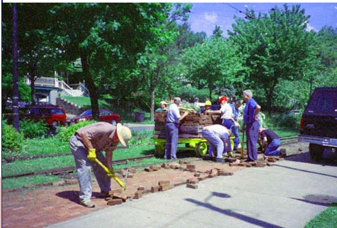
D-Day (May 31st)— Here’s the Tuesday crew taking up the platform pavers in front of the Linden Hills station.
