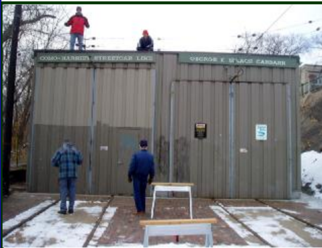
Men at work! Aaron Isaacs (left) and Russ Isbrandt are on the roof while on the ground are Phil Settergren (L) and Keith Lindberg after installing the sign on the front of the Isaacs carbarn. (John Prestholdt photo)
