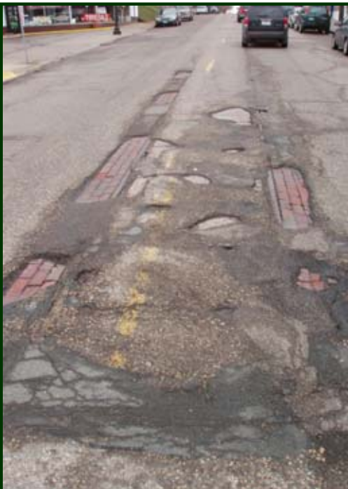
A sure sign of spring! After the spring freezes and thaws are over out comes the evidence that at one time dinosaurs roamed the land. Here we see two rails peeking through the broken pavement at the intersection of Xerxes Ave. and 50th St., about a mile away from our CHSL line. This is the leg of the wye where the OAK-XERXES cars reversed course for the trip back to downtown Minneapolis. (Aaron Isaacs photo)
