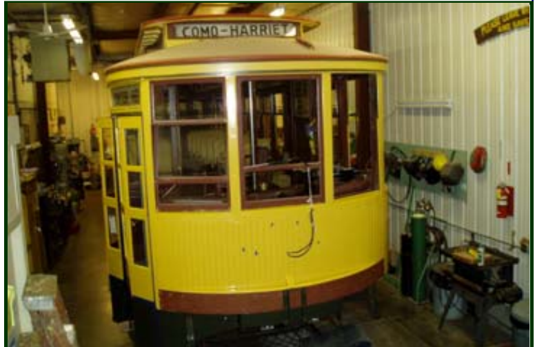
Almost Finished! The rebuilt front end of No. 1300 is almost done. Still to come is installation of the "golden glow" headlight and the rubber bumper on the front end. (John Prestholdt photo)
