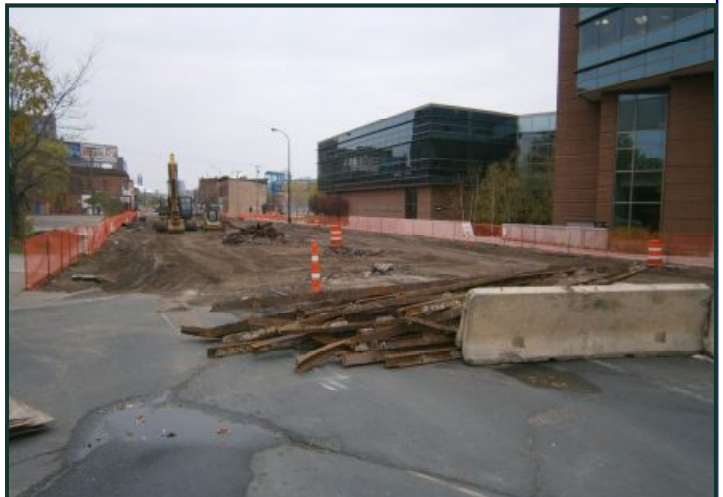
Dig we must! It's not only University Avenue where you can see old streetcar rails being unearthed during street construction. Here we see Riverside Avenue in Minneapolis being rebuilt and what do they find? Tons of old TCRT 90-pound "T" rail. Not much good except to the scrapper. (Photo by Aaron Isaacs)
