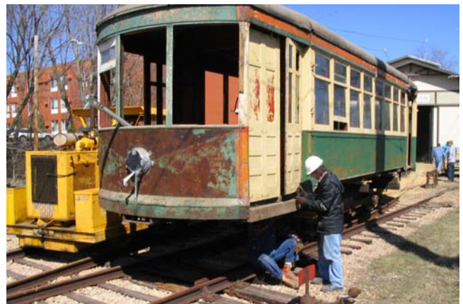
Here's a close-up of Winona No. 10. Note the "traction orange" paint and red stripe on the corner post and the "hourglass" showing thru the rust on the end. The orange body with red stripe was the last paint scheme used on Winona No. 10--the hourglass disappeared in the early 1930s. That's Ken Albrecht with his legs sticking out from under No. 10 while Mike Miller (standing) adds some encouraging words. (Tom Fairbairn photo)
