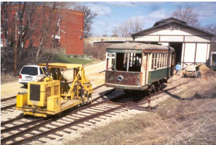
The cars on tracks 1 and 2 had to be moved out to allow the contractor to relocate track 1 inside the ESL carbarn. In this photo taken on April 1, 2004 you see Winona No. 10 outside the carbarn for the first time in perhaps 3 or 4 years. (Jim Vaitkunas photo)
