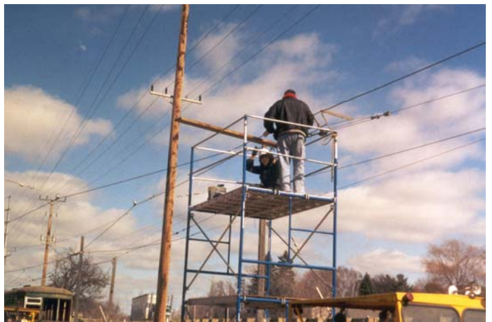
Overhead Wire work! Scott Heiderich and Mike Miller are up on the tower car working on the ESL overhead. (Jim Vaitkunas photo)
