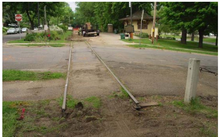
It didn't take the contractor long to take up the old rails and ties. Here's a photo of the 42 nd Street crossing taken on June 3 rd . ( Wendy Dunham photo )
