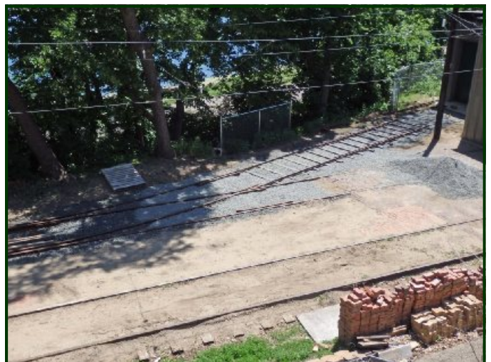
(Left & Above) Still some more work needs to be done on the track in the shed, but it's looking good.
