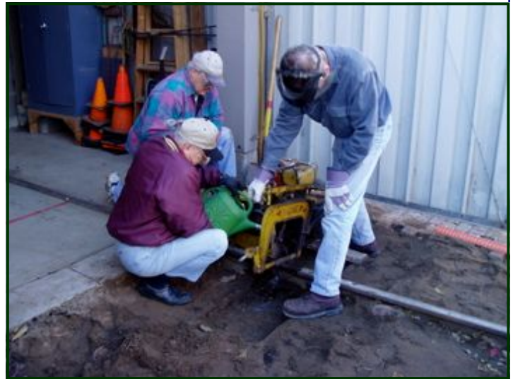
Both rails of the Isaacs car barn’s “ready barn” track had to be removed and the ties taken up so the contractor could dig a trench to install the water pipe. Here you see (left to right) John Prestholdt , Dennis Stephens and Keith Anderson mounting the power rail saw so the rail could be cut. ( John Prestholdt photo )
