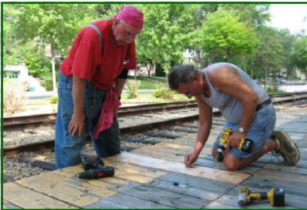
Platform Repairs. Jim Otto (left) and new Volunteer Bob Smith (right) are seen here replacing yet another rotten board on the Linden Hills station's platform. (John Prestholdt photo)
