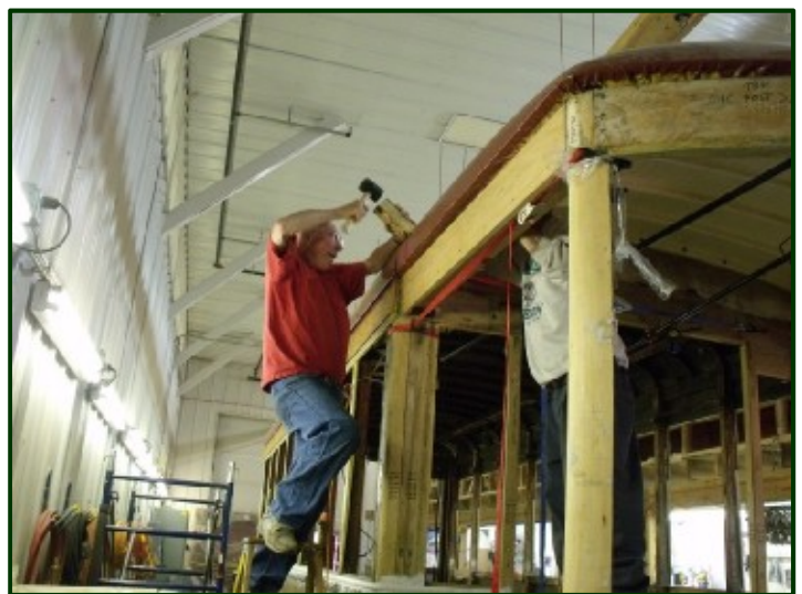
The roof has now been pushed to the main passenger compartment roof. It's a very tight fit and after being "greased" with Vaseline, Ken Albrecht is "persuading" the platform roof to fit under the main roof. Tom McGruder is on the right helping to steady things. (Jim Vaitkunas photo)
