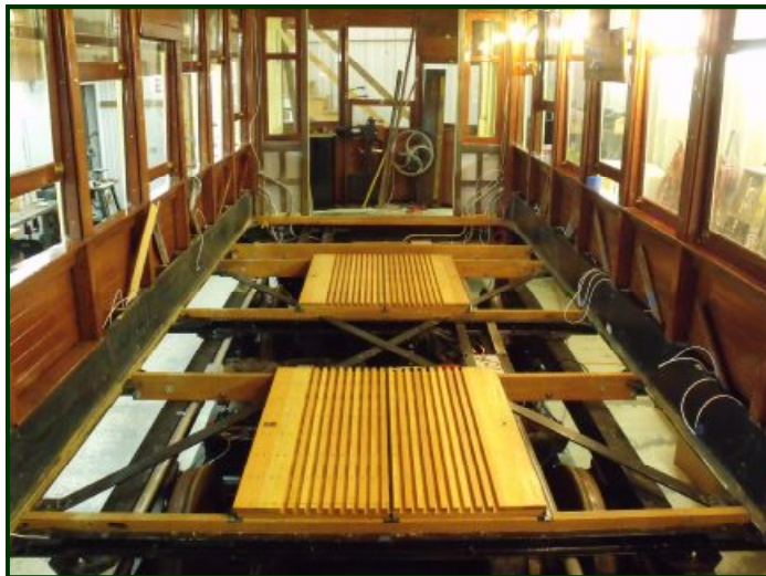
The two floor pieces show in this photo are removable so our shop volunteers can gain access to the motors and air compressor. The rest of the floor will be permanently installed once all underfloor work is completed.
