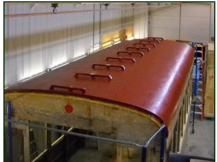
Here's the freshly painted roof with the trolley board cleats installed on the roof's centerline. Two trolley boards will be attached to these cleats and in the middle the trolley pole base will be attached to the trolley boards. Winona No. 10 had only one trolley pole so at the end of the line, the pole had to be swung around. (Howie Melco photo)
