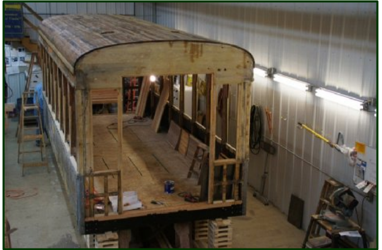
This photo was taken in April, 2011. Roof repairs are complete and the shop guys are ready to put on the canvas. The roof boards were first sanded and then several coats of boiled linseed oil were applied. (Dick Zawacki photo)
