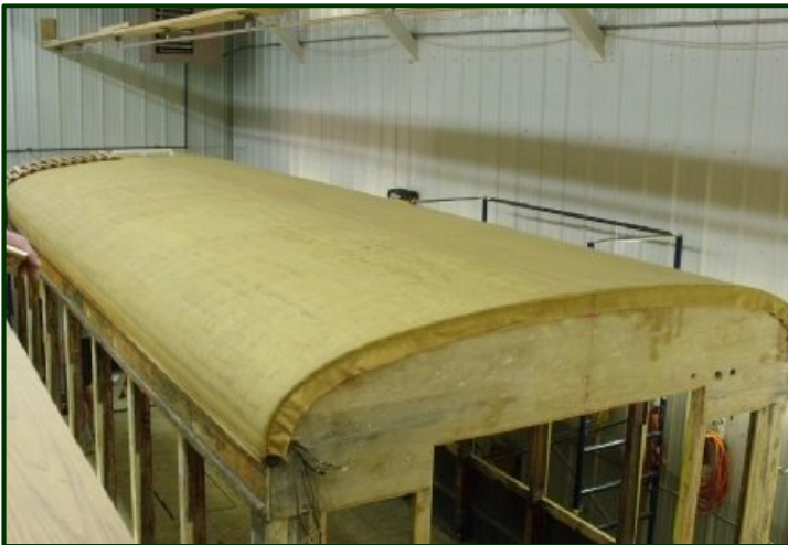
The canvas roof is on, stretched tight and then saturated with several coats of boiled linseed oil. It's now ready for the color coat and installation of trolley board cleats. (Jim Vaitkunas photo)
