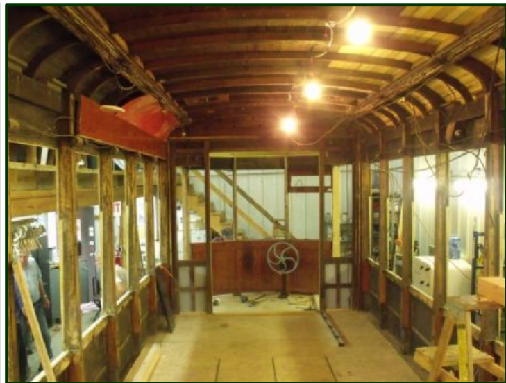
Here is the "bare bones" look of the streetcar at the moment. It looks like the guys have put up some of the interior shown on the upper left to see how things will fit. The floor is also temporary to allow for later under-floor work as mentioned above. (Jim Vaitkunas photo)
