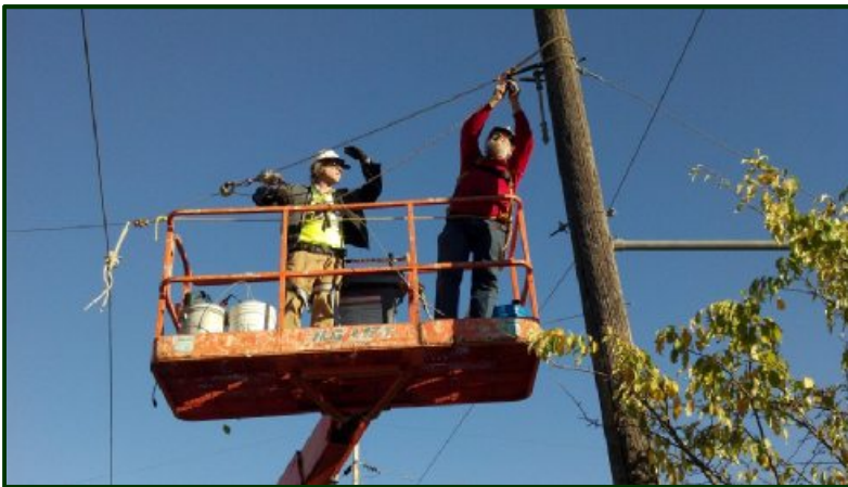
Mike Miller (Left) and Scott Heiderich work on the overhead span wire.
