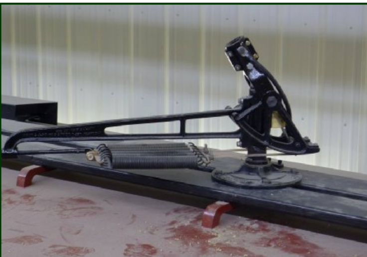
Here's the trolley pole base just installed on the roof's trolley boards. This photo was taken a few hours after the photo on the right. Dennis Stephens worked on rebuilding the trolley base.
