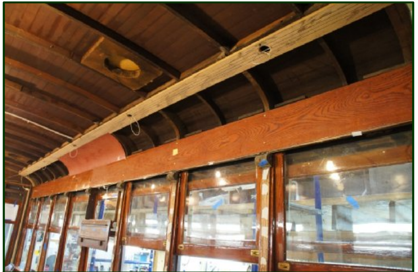
Interior lighting circuit wiring is also roughed in by Mike and Scott.
