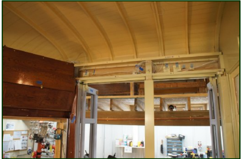
Wiring for the light bulbs over the main doors is roughed-in right now. Mike Miller and Scott Heiderich are working on the interior wiring.
