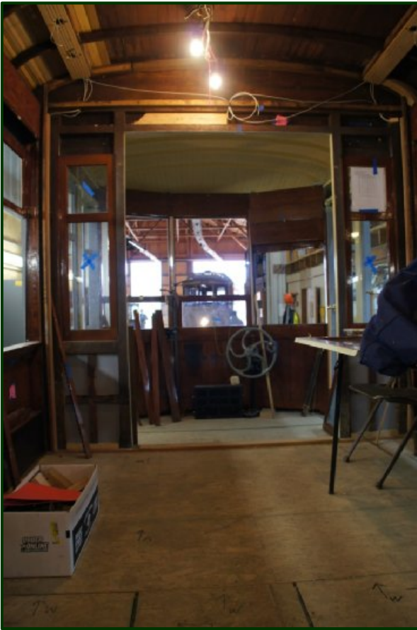
Other than missing controllers and air brake stands, the front platforms are nearly complete. Pipe railings will also be installed on each platform to control passenger flow.
