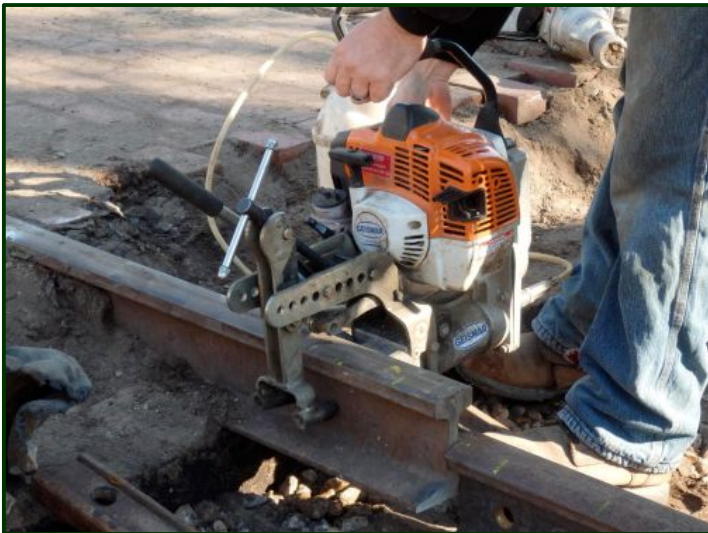
Here one of the Railroad Specialties workers is drilling a bolt hole.
