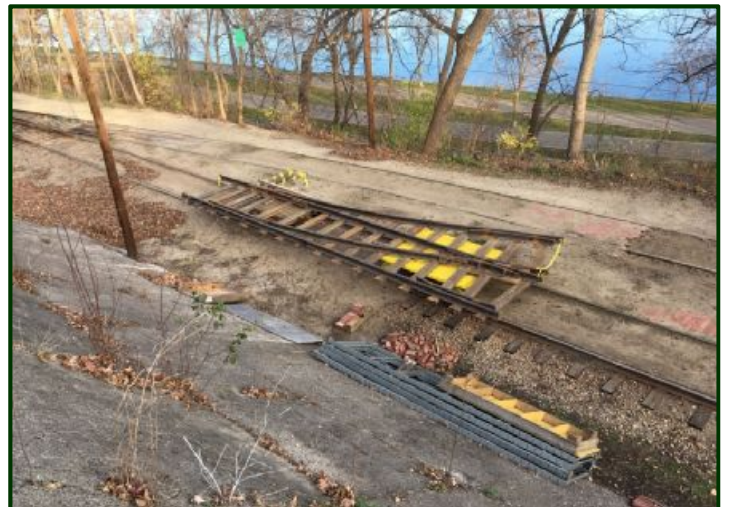
The switch sat in front of the Isaacs car barn waiting for installation by Railroad Specialties.
