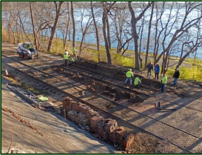
On November 16 th , the Railroad Specialties crew arrived and started work to remove the carbarn lead track where the speeder shed switch will go.
