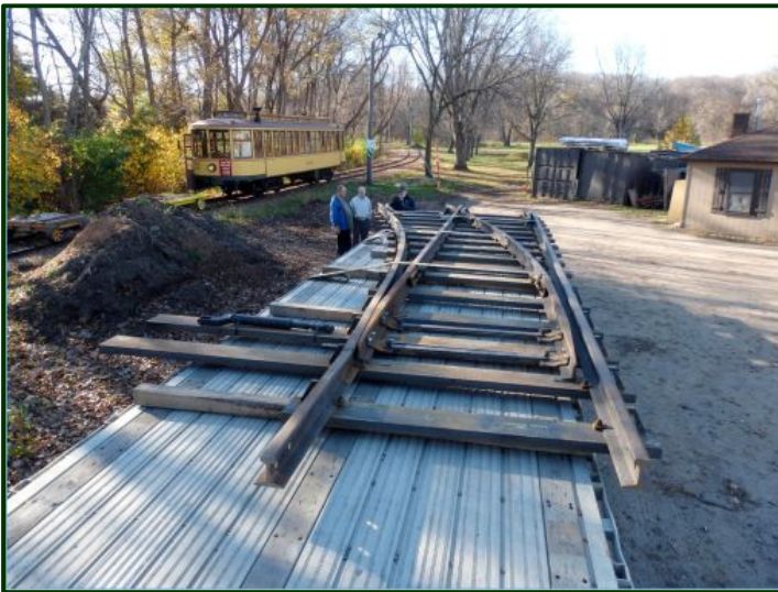
On November 9 th , the flatbed from Harmer Steel delivered the switch to the Park Board's maintenance area adjacent to Lakewood Cemetery and Lake Calhoun, which was the best place to unload and temporarily store the switch.
