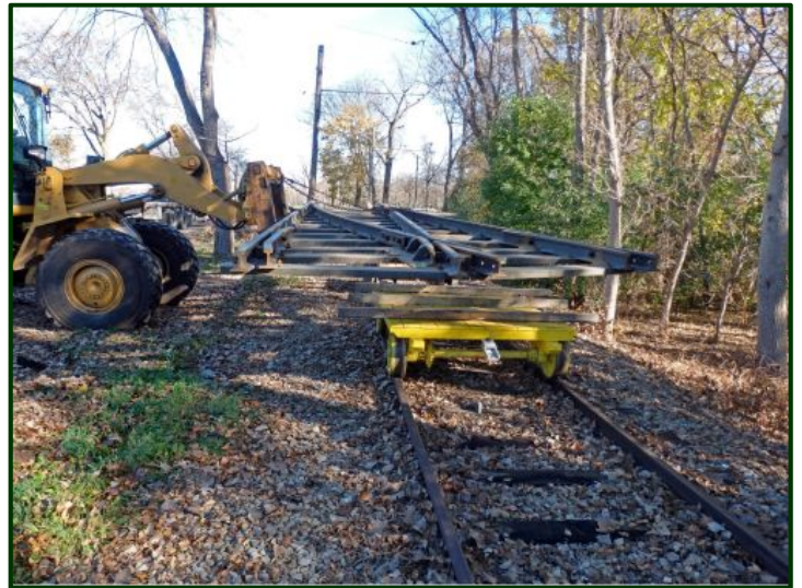
A heavy-duty forklift courtesy of the Park Board put the switch onto two maintenance flats for transport up to the Isaacs Car barn and Shop when it's needed for installation. Until then, the switch remained there to wait for the track crew to install it.
