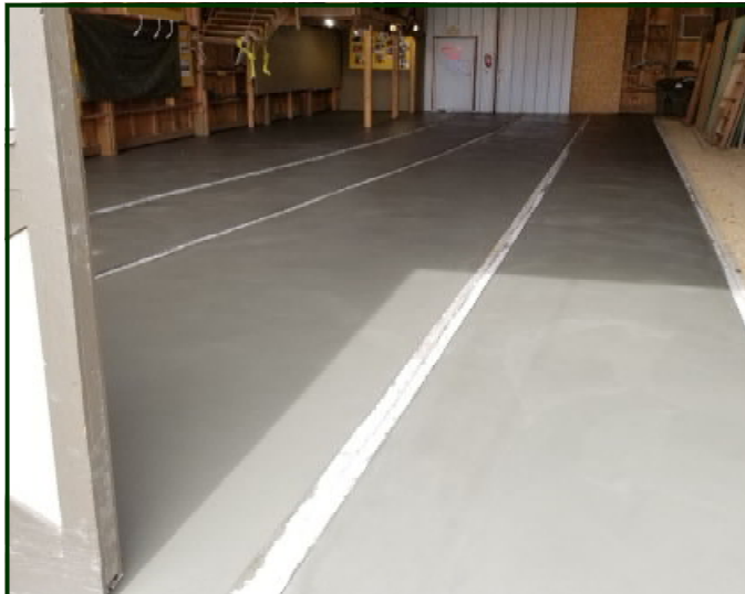
In May, 2017 a concrete floor was installed in the Excelsior car barn which greatly improved that building.
