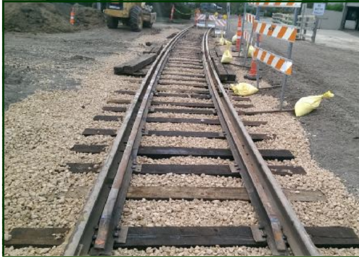
In 2014, sewer work on Morse Avenue at ESL resulted in a new and improved crossing for our Excelsior Streetcar Line.
