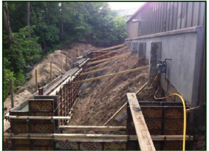
Work started on the Isaacs car barn addition in 2015. This photo shows the foundation being constructed. The addition was dedicated in 2016.
