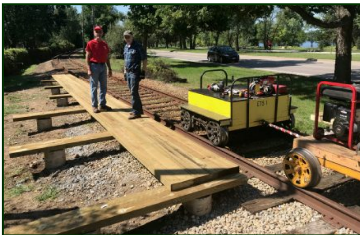
The new Lakewood Cemetery platform is coming along. Here's Keith Anderson and Bill Arends working on the partially completed deck.
