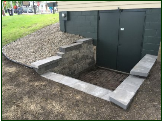
As reported by Aaron Isaacs on page two, we had a contractor come and re-do the step well and steps to the Linden Hills station's basement entrance. They did a great job in improving both the appearance and access to the basement, and gave us a very favorable price for the work. (Aaron Isaacs Photo)
