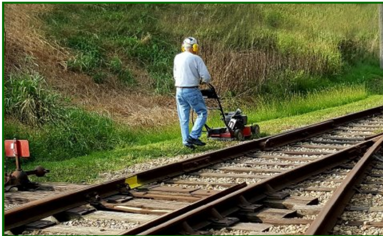
While COVID-19 has caused ESL's car barn and shop work to cease, the outside work still needs to be done. Here we see Ken Blake cutting the grass on the south side of the ESL car barn tracks. (MSM photo archive)
