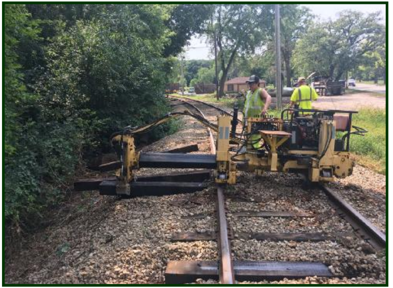
Railroad tie extractor and new tie inserter at work. (Photo by Aaron Isaacs)
