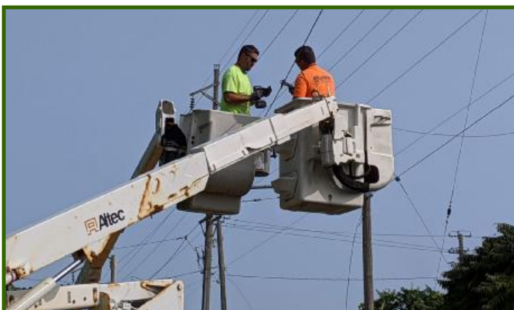
The first pull-off is clamped to the trolley wire. The wire to the backbone will then be tightened to pull the trolley wire closer to the center of the track, but about six inches off the center-line. (Jim Vaitkunas photo)
