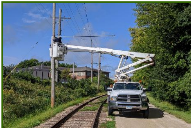
Killmer's crew started their work on 9/9/2020 on the west end of ESL. Here, the crew is installing a backbone wire. Two pull-offs will be installed between each pair of support poles. (Jim Vaitkunas photo)
