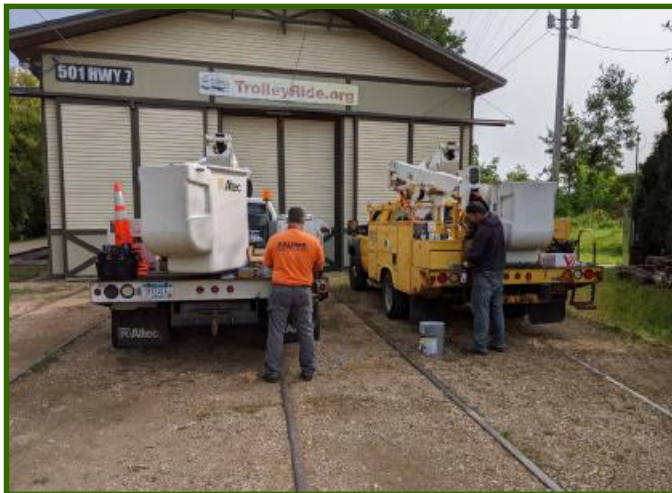
After the backbones were installed, the crew pre-assembled the pull-off insulators, wire and clamps. The crew Foreman was Jeff Tuccitto (L) and Graham Harding (R). (Jim Vaitkunas photo)
