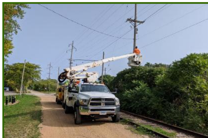
The Killmer crew started installing the pull-offs at the east end of ESL. (Jim Vaitkunas photo)
