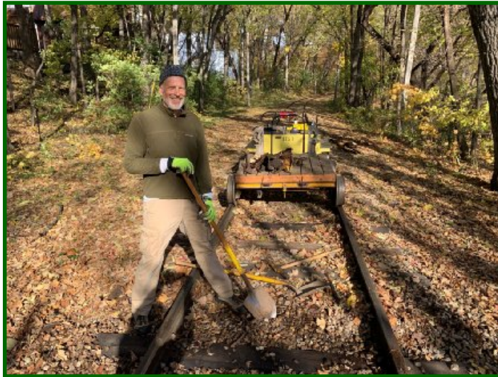
What better way to spend a fall afternoon than to replace bad cross-ties at CHSL! Here's CHSL track Foreman Miles Anderson and Keith Anderson (the photographer) who replaced 10 ties in a morning.
