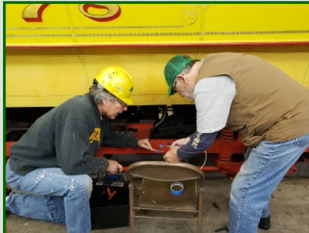
Carl Floren (L) and Scott Heiderich are seen here working on an upgrade to Duluth No. 78's ditch lights.
