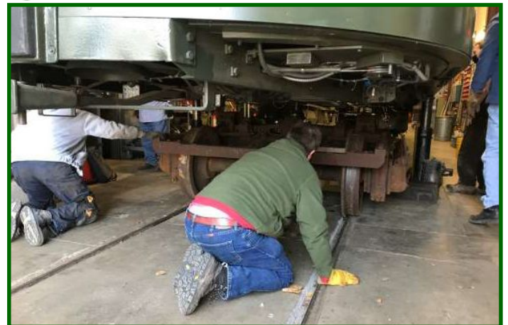
When the shop truck from IRM arrived, it replaced 1239’s front truck. This allowed work to begin on dismantling the old truck. Here we see Karl Jones (L) and Ben Franske positioning the shop truck under the front end of No. 1239.
