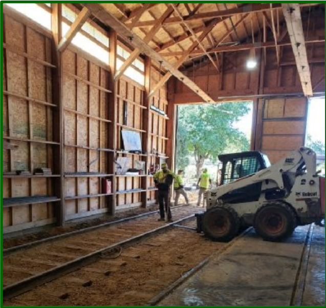
With everything cleared out from track #3, local railroad construction company Railroad Specialties Inc., began the process of aligning the track with the center of door #3. With the track now properly aligned, all the cars at ESL can safely access track #3. The next step is to finish the concrete floor around track #3, which was done in December 2022.
