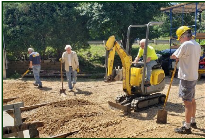
Completing the gravel work around the new concrete apron in front of the ESL car barn doors. (L to R) Tom Heimer, Michael Kimitch, Howie Melco and Carl Floren. (Karen Kertzman photo)
