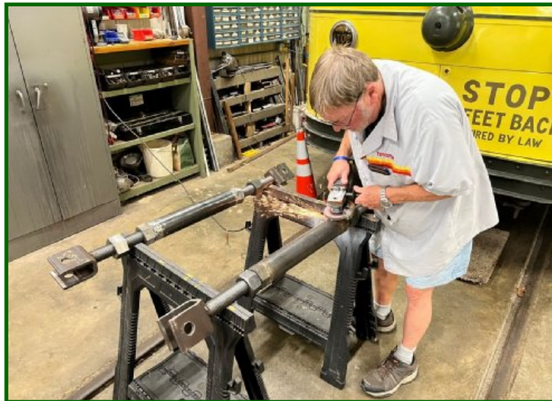
(Above) Work on rebuilding TCRT No. 1239's truck is progressing. Here we see Tom Schramm working on gringing out rough spots on two of the brake slack adjusters. (Aaron Isaacs photo)
