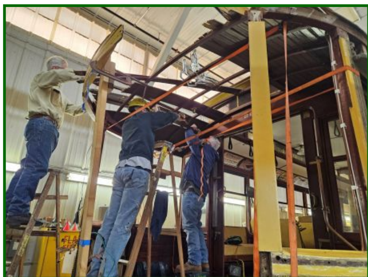
(Above Right) Dick Zawacki , Howie Melco and Tom Heimer are discussing strategy for DSR No. 265's rear vestibule roof repair. (Right) Tom Heimer , Carl Floren , and Scott Wardrope removing damaged roof boards. (Both photos by Karen Kertzman)
