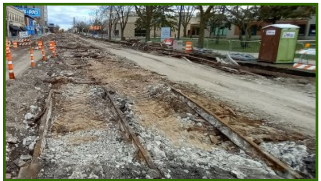
Hennepin Avenue in South Minneapolis is being rebuilt and look what they found. Como-Harriet cars once ran on these rails. (Photo by Nick Mainguy)
