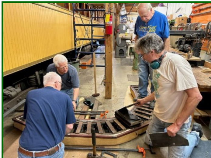
It's a team effort getting the rear bench seat ready for installation in DSR No. 265. Scott Wardrope, Howie Melco, Carl Floren, and Dick Zawacki (standing). (Photo by Jerry Draeger)
