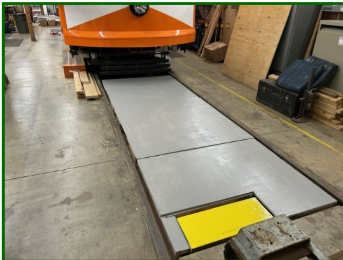
New Pit Covers. ESL's shop area has a pit and new covers have been fabricated as an important safety measure. The pit covers are reinforced so a person can walk on them. The yellow thing is the top of the steps down into the pit. (Photo by Karen Kertzman)
